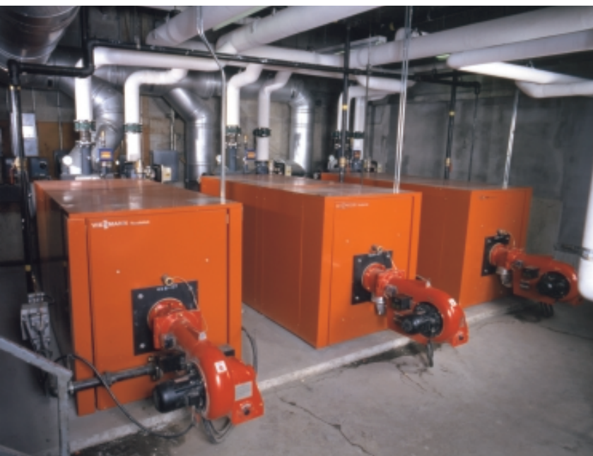
Viessman high efficiency boilers installed as part of retrofit program
