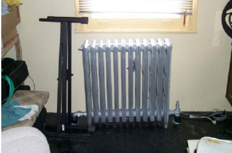
Figure 5-1 Cast Iron Radiator, Centre Calixa-Lavallée
