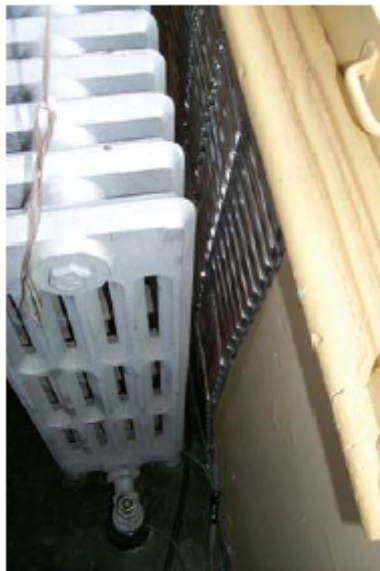
Figure 5-3 Reflector Panels behind a Radiator
