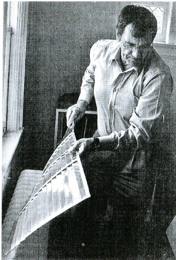
Frank Snyder installs heat reflector panels behind a radiator in a Toronto home. FERNANDO MORALES/THE GLOBE AND MAIL
